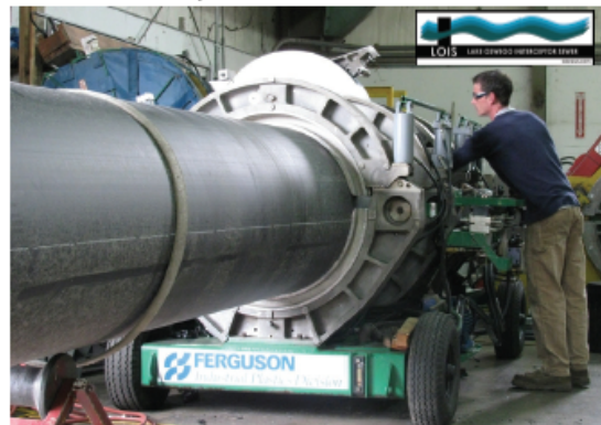
Pipe fusing equipment to be located at McVey site.
