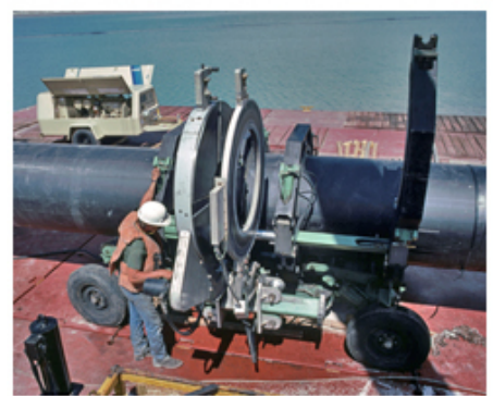
Pipe fusing will begin from the dock near Oswego Dam in the fall.
