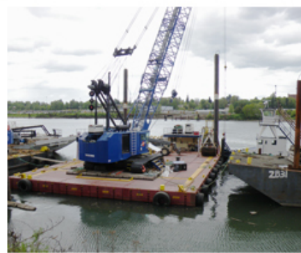
Equipment similar to this crane and barge will appear on the lake in coming months.
